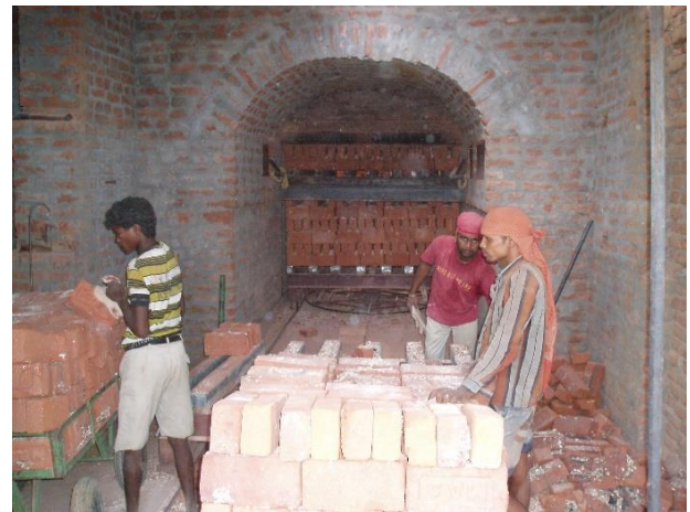
FIGURE 38 INSIDE A VSBK UNIT
