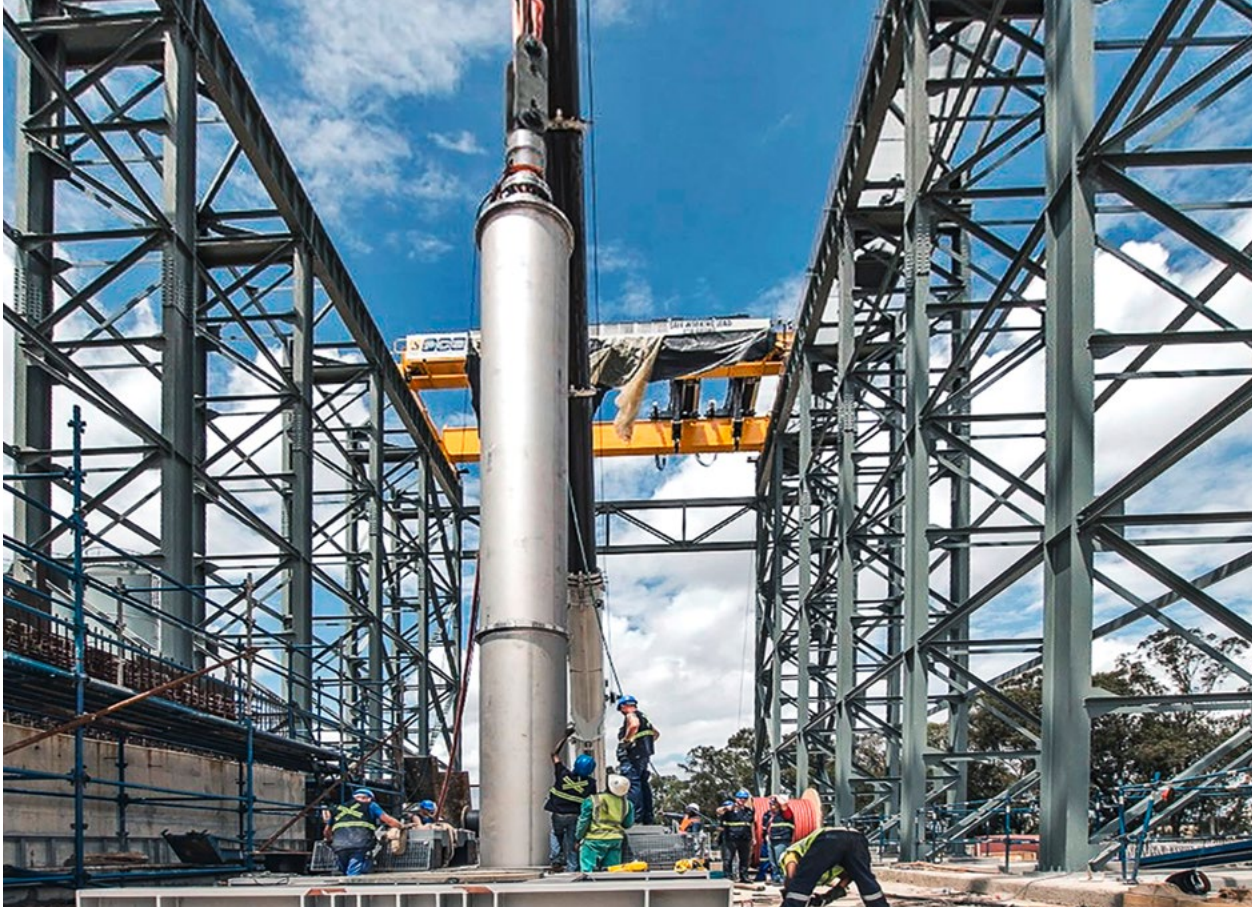
Figure 2: Installation of one of the ANDRITZ pumps
