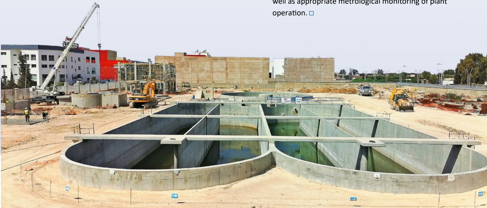
Figure 1: Aeration basins under construction at the industrial wastewater treatment plant in Nouaceur, Morocco
