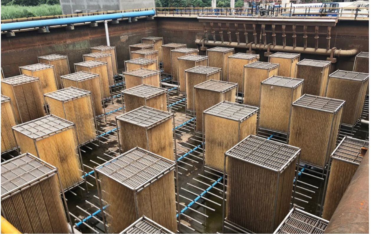
Figure 1: One of six SBR basins with Biocurlz cages and fine bubble tube aerators
