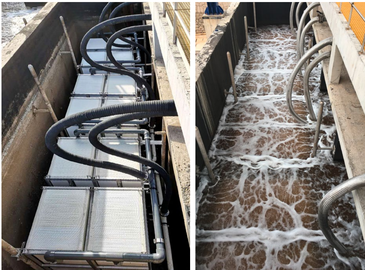
Figure 1: Submerged membrane modules after installation (left) and in operation (right)
