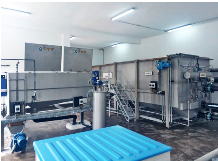
Figure 1: Space-saving installation – Flomar® flotation for wastewater pre-treatment and screw press for sludge dewatering in a fish factory in Morocco
