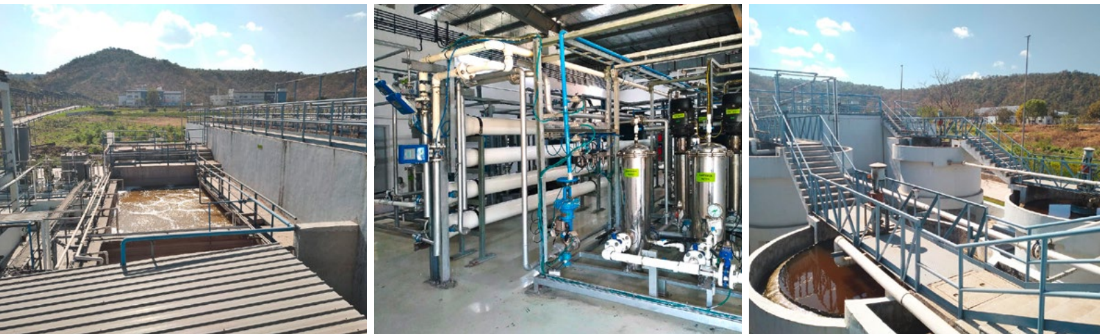
Figure 2: 8.3 m 3 /h SUFRO ® plant near Mumbai, India – Biological cleaning (left) Reverse osmosis (centre) Secondary clarifier and ultrafiltration tank (right)
